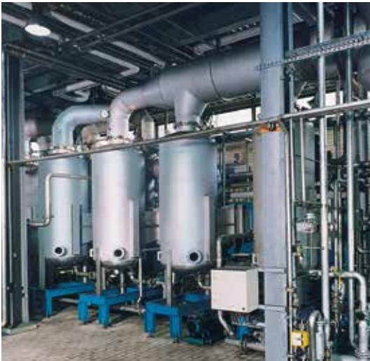
Multiple-effect plate evaporation plant for fructose. Evaporation rate: 16 t/h
