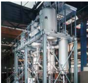
3-effect circulation evaporation plant for glycerine water. Evaporation rate: 3600 kg/h
