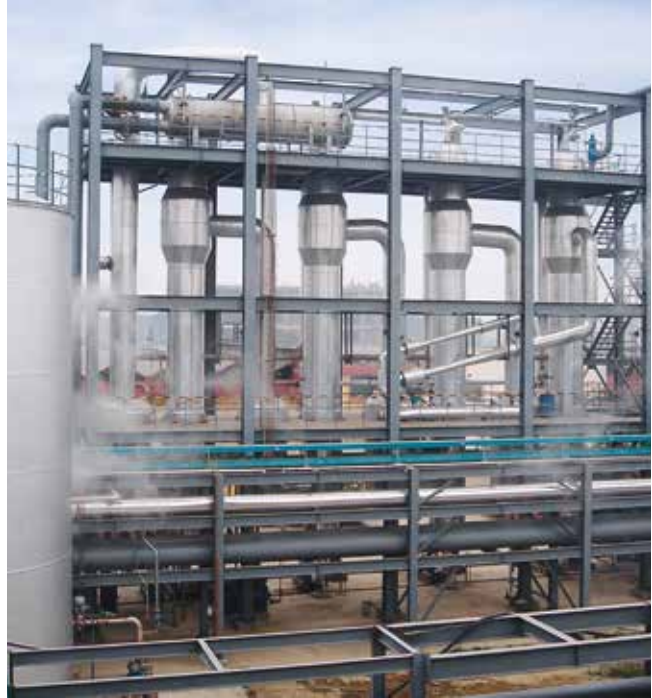
4-effect falling film evaporation plant heated by thermal vapor recompressor for lysine solution Evaporation rate: 47 t/h
