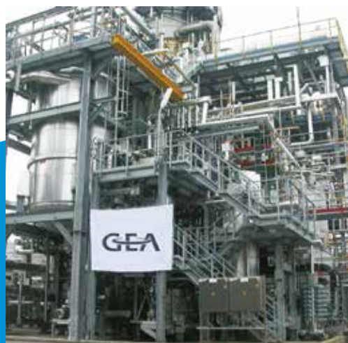
Melt crystallization plant for benzoic acid purification
